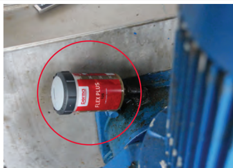
Bearing lubrication on a pump
