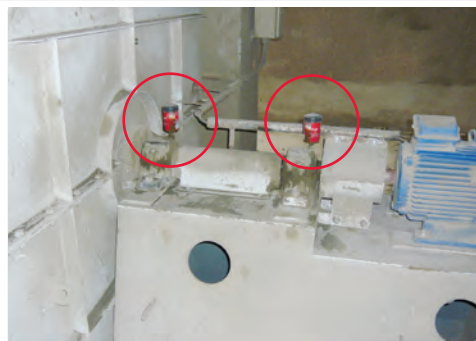
Lubrication of pillow block bearing on a fan drive shaft
