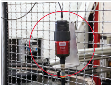
Automatic lubrication of a sliding guide
