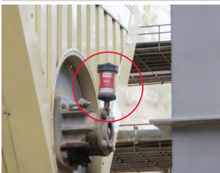
Flange bearing lubrication on the dedusting trough screw conveyor
