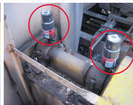
Lubrication of a fan drive shaft bearing
