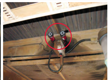
Fin fan lubrication in a heat exchanger
