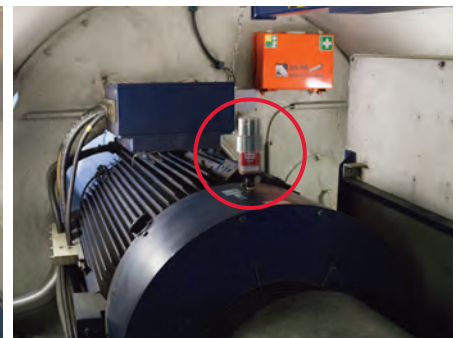
Automatic relubrication of the generator bearing
