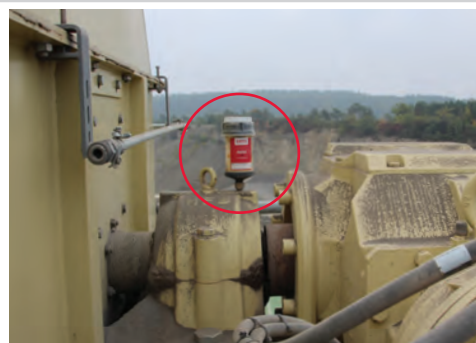
Roller bearing lubrication on the hot vertical bucket conveyor
