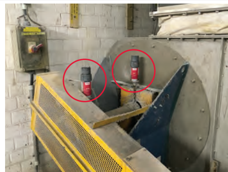
Pillow block bearing lubrication on a fan
