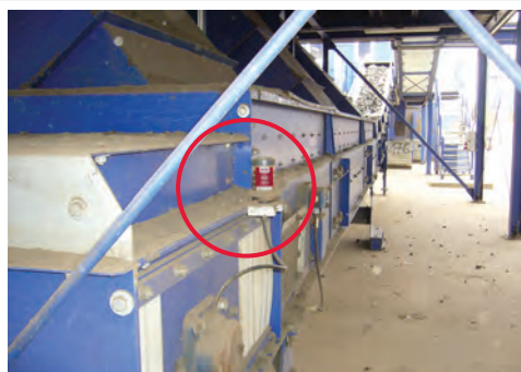
Flange bearing lubrication on a conveyor
