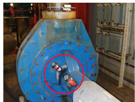
Drive shaft lubrication on a pump
